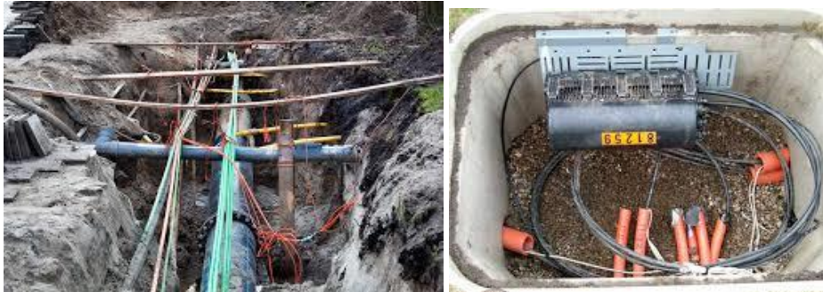
Fig: picture indicating underground fiber optic installation
