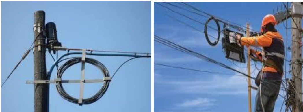
Fig: Picture indicating Aerial installation of fiber optic network
